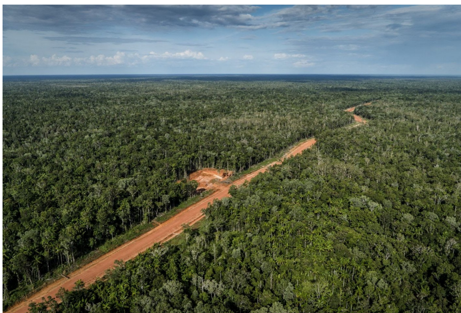
View over the MIFEE highway cutting through dense forest in Merauke, built around 2012. Photo taken by Ulet Ifansasti for Greenpeace
